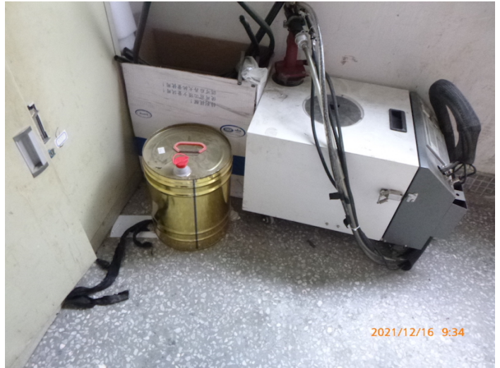
NC: no secondary container provided for chemical
