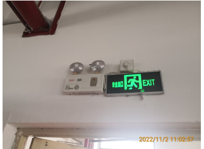
Exits sign and emergency light
